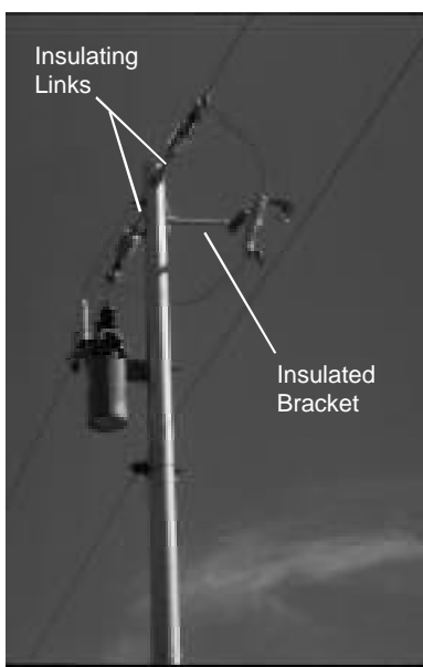
Photo 6. Steel single-phase double deadend pole with insulating links to achieve 300kV BIL.
