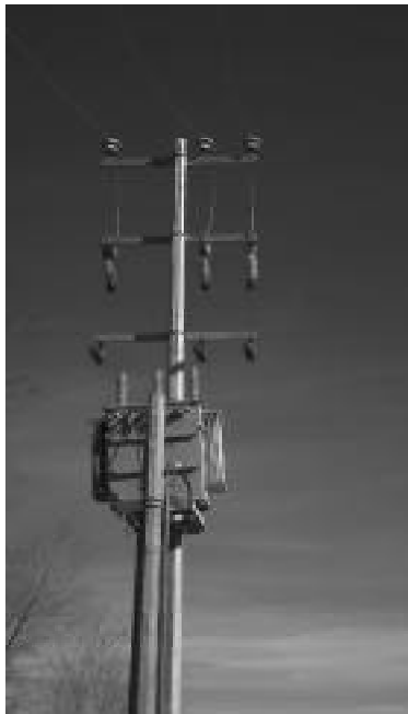
Photo by Cynthia Melcher Photo 3. Concrete pole associated with raptor electrocutions in San Pedro, Mexico.
