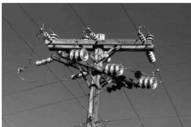
Photo 7. Deadend structure with inadequate separation between jumper wires.
