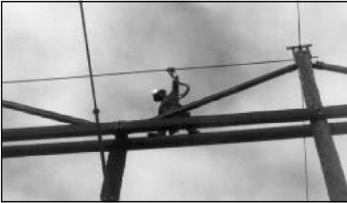
When working on a live line, linemen prefer to work inspection or replacements with wood poles over conductive steel poles which require additional phase-to-structure insulation.
