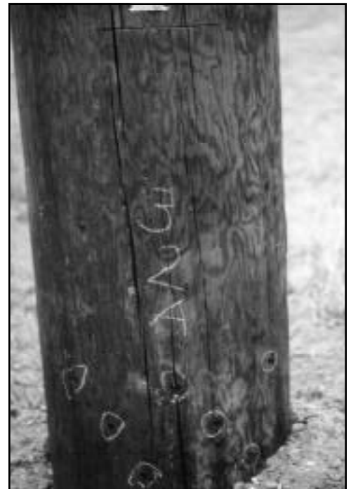
Typical boring patterns are 2 feet above groundline and 3-4 feet below.
