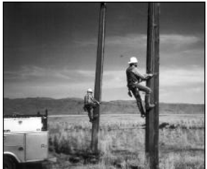
Linemen prefer to work with wood poles as climbing using gaffs or hooks is easier and allows better positioning on the pole.
