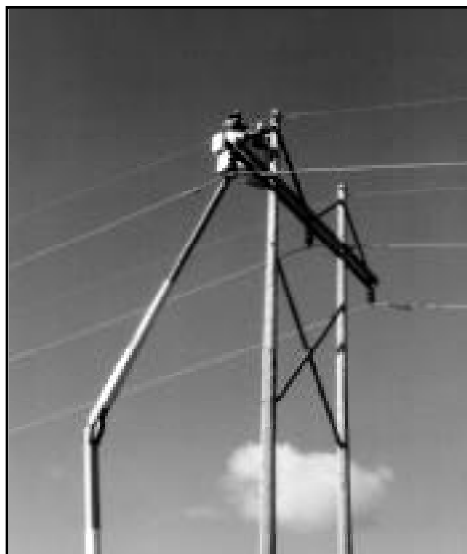
Field modifications can easily be made to wood poles using simple-to-use utility drills.
