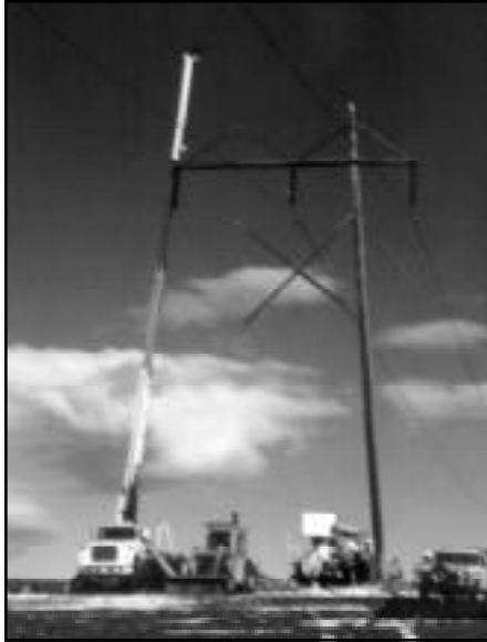
For distribution and small-to-medium transmission poles, a line bed can be used to dig the foundation and lift the pole into position.
