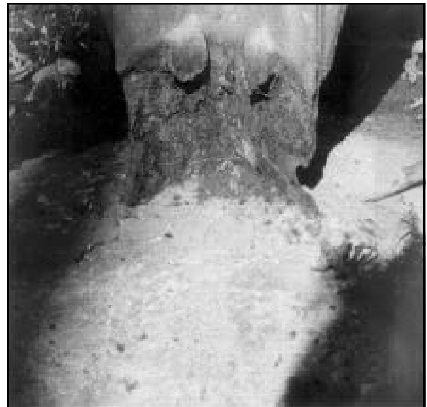
Weathering of steel poles can compromise the protective coating causing pitting or flaking of the steel material.
