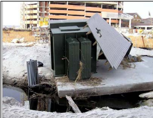
Figure 6: Destruction of Pad-Mounted Transformer Caused by Tidal Surge And Beach Erosion from Hurricane Ivan (2004)
