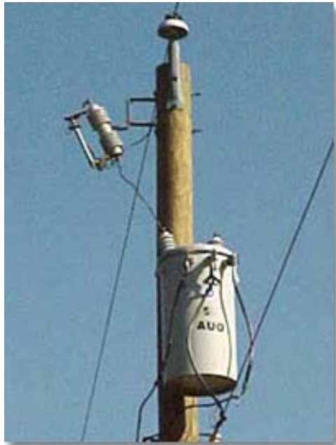
Figure 2: Typical Pole-mounted Transformer
